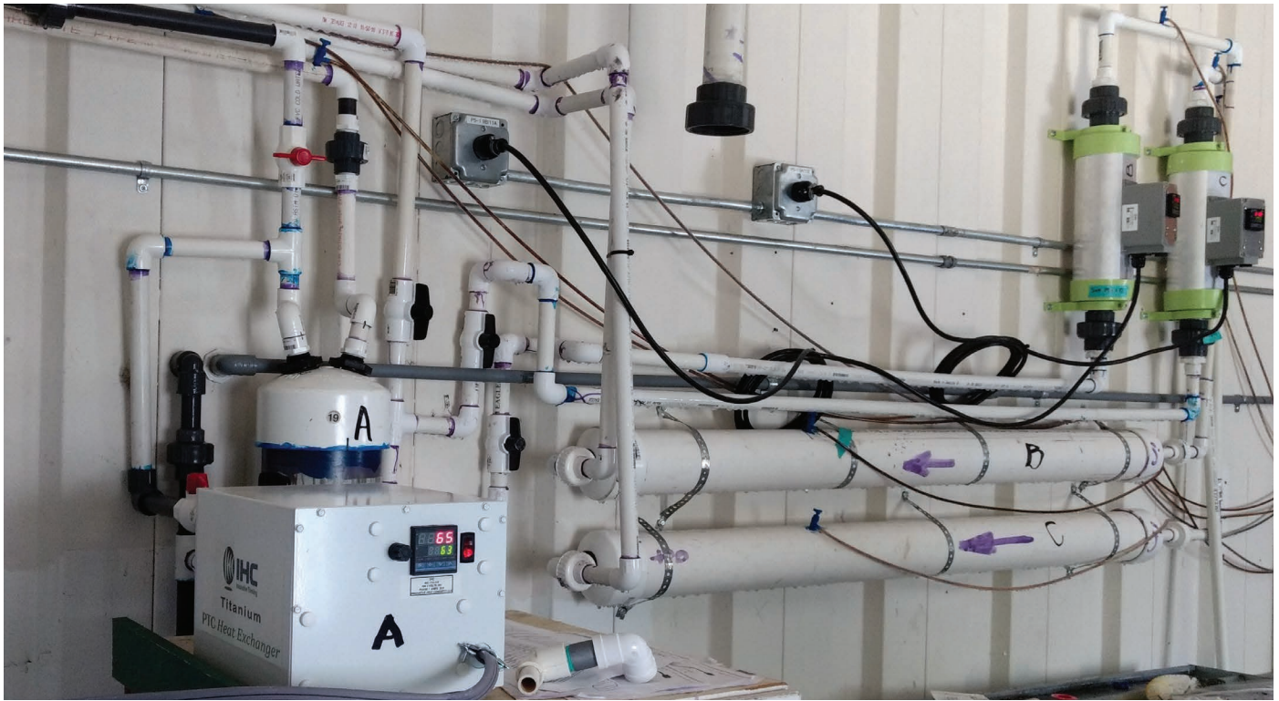
FIGURE 1. In-line heaters with mixing cells were used to warm three of the treatment temperatures above the ambient groundwater temperature (Photo: James Barron).
